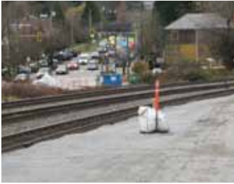
Pre-load in preparation for the relocation of rail lines to make room for the Evergreen Line guideway in Port Moody.
